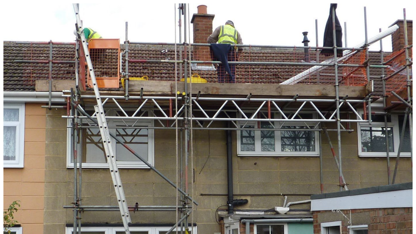
An example showing acceptable edge protection. HSE inspectors would expect to see this standard of protection during solar panel installation
