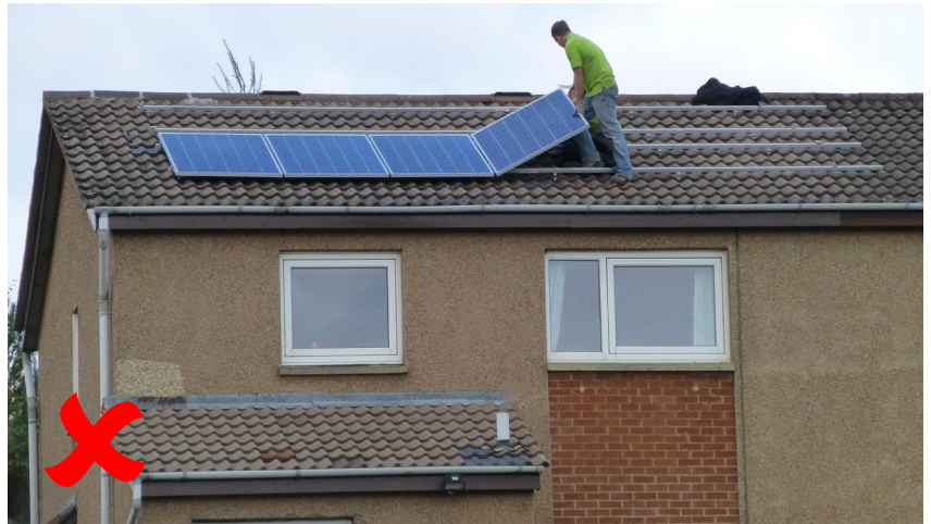
An example of completely unacceptable installation work practices that could easily result in death or serious injury. Unsafe work at height like this would normally lead to immediate enforcement action by HSE inspectors
